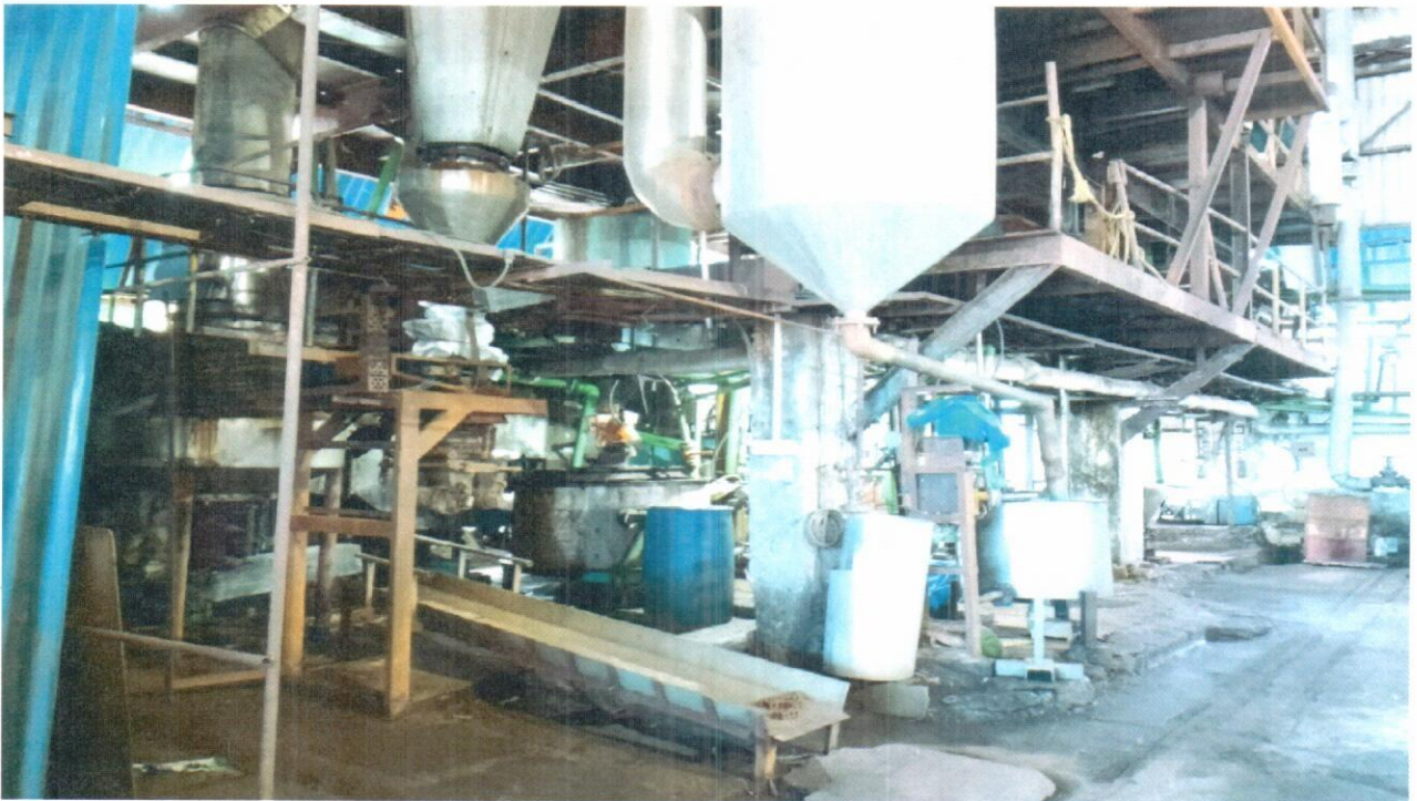
Sodium Sulphate Evaporation Plant for Process water treatment
